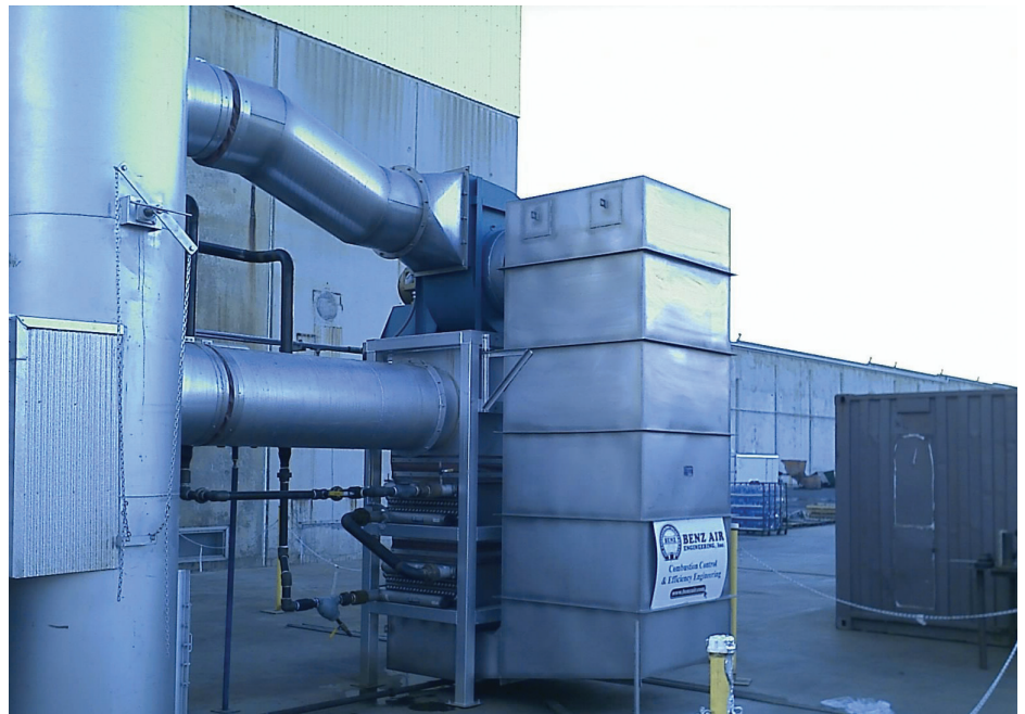
Del Monte Foods' Super Boiler flue gas condensing heat exchanger has a boiler fuel-to-steam efficiency exceeding 93 percent.
